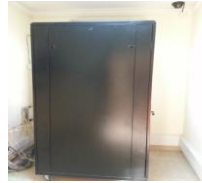
Secure data room with rack space for communication equipments
