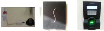
Access control and monitoring at main entrance, each work room and all access points
