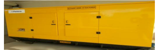
Generator for uninterrupted power
